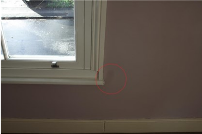
Bedroom 1 - damp by window
