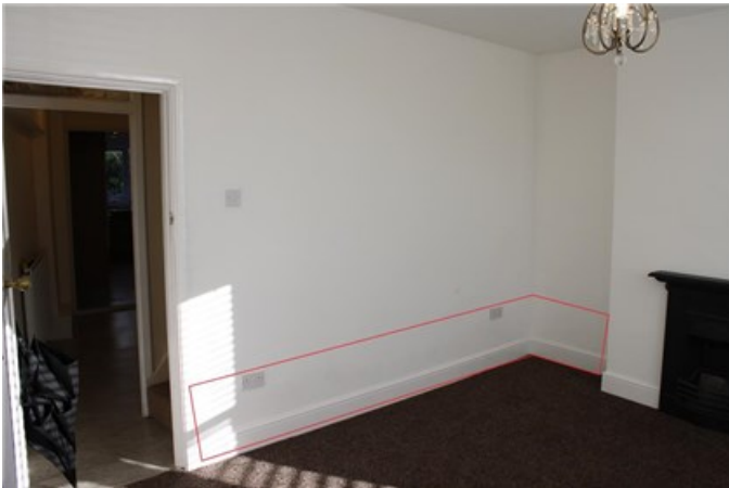
Lounge - rising damp to internal and party walls
