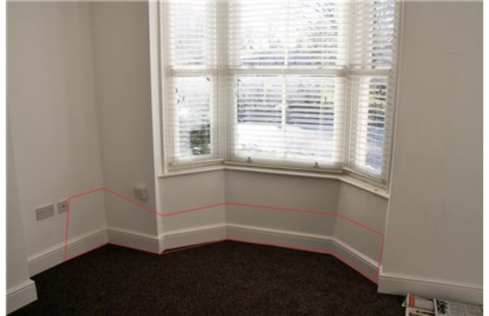
Lounge bay and party wall with rising damp
