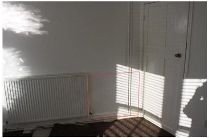
Lounge side wall - area of damp
