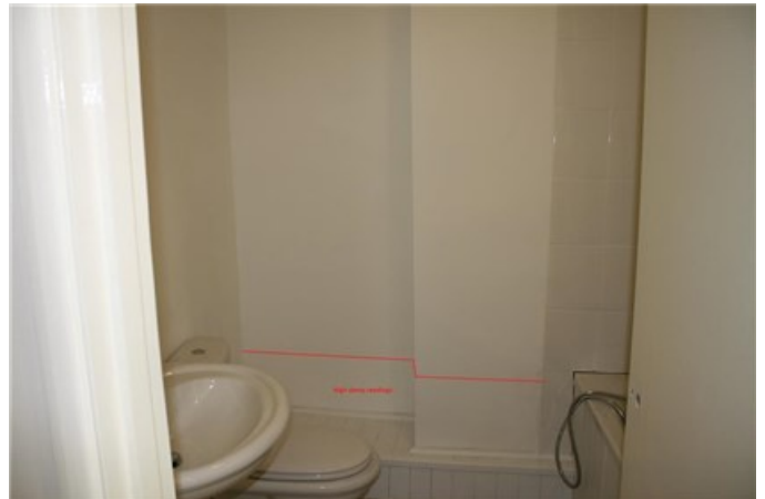
Bathroom - damp in the party wall and chimney breast
