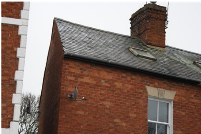
Gable wall - leaning out slightly at top
