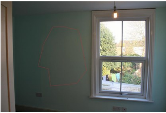
First floor rear wall - medium levels of damp detected
