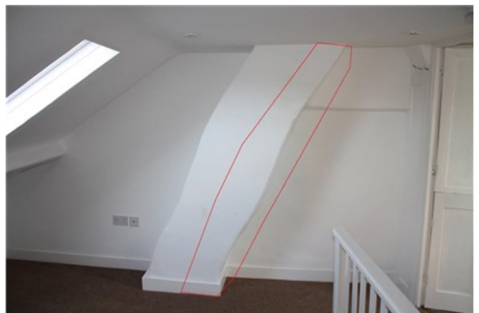
Rear 2nd floor bedroom - damp in chimney breast
