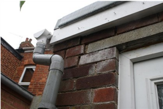
Kitchen rear wall - mortar missing
