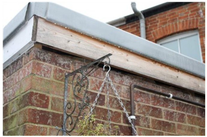
Flat roof - gap can be seen where edge isn't finished
