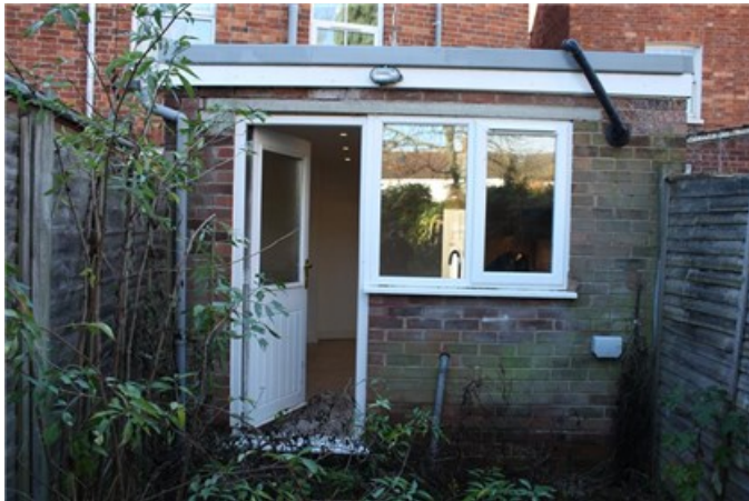
Rear wall - brickwork looks damp
