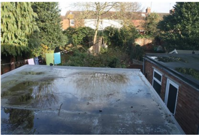
Flat roof to kitchen - rainwater is pooling
