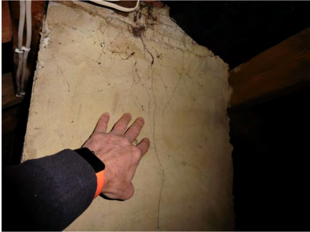
Light cracking of the right side chimney breast in the roof space
