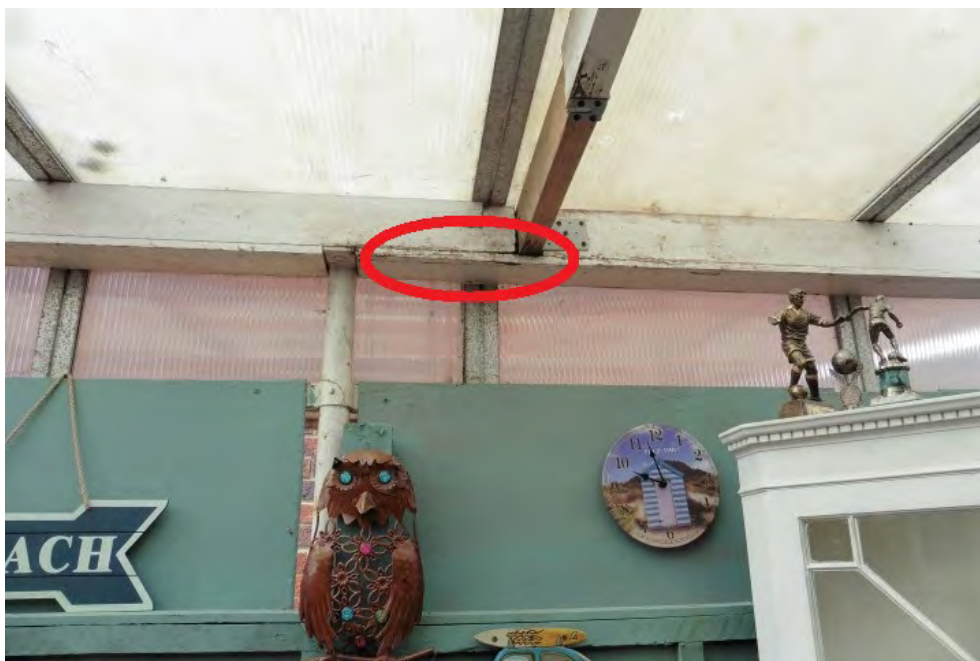
Possibly rotten timbers in the lean-to
