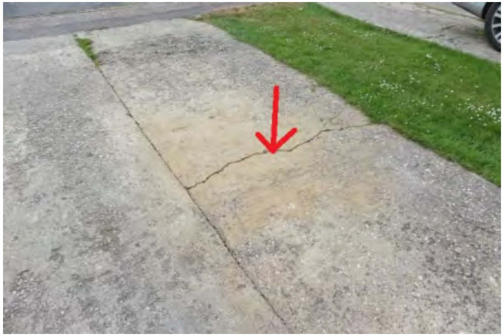
Cracking in the front drive
