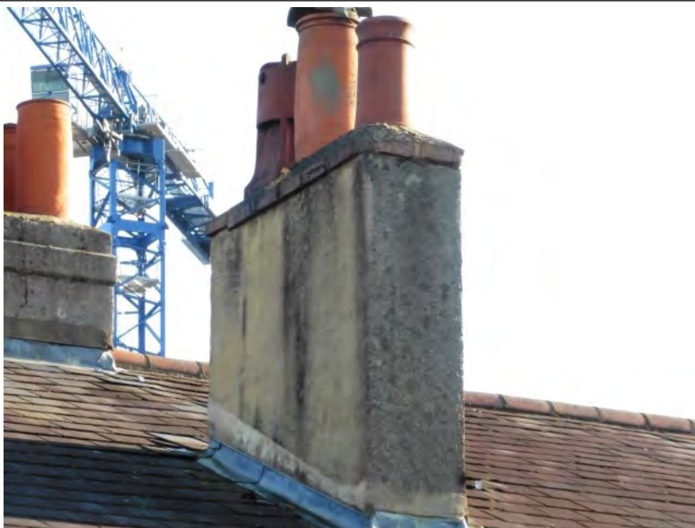
Rear stack viewed from the rear
