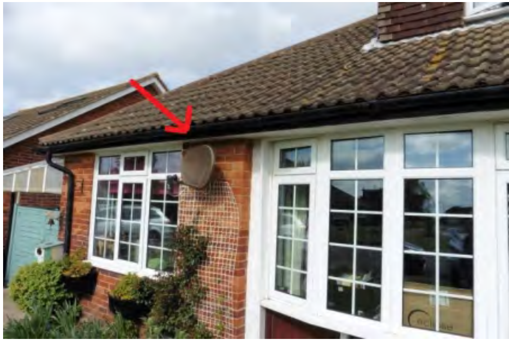
Sagging gutter at the front
