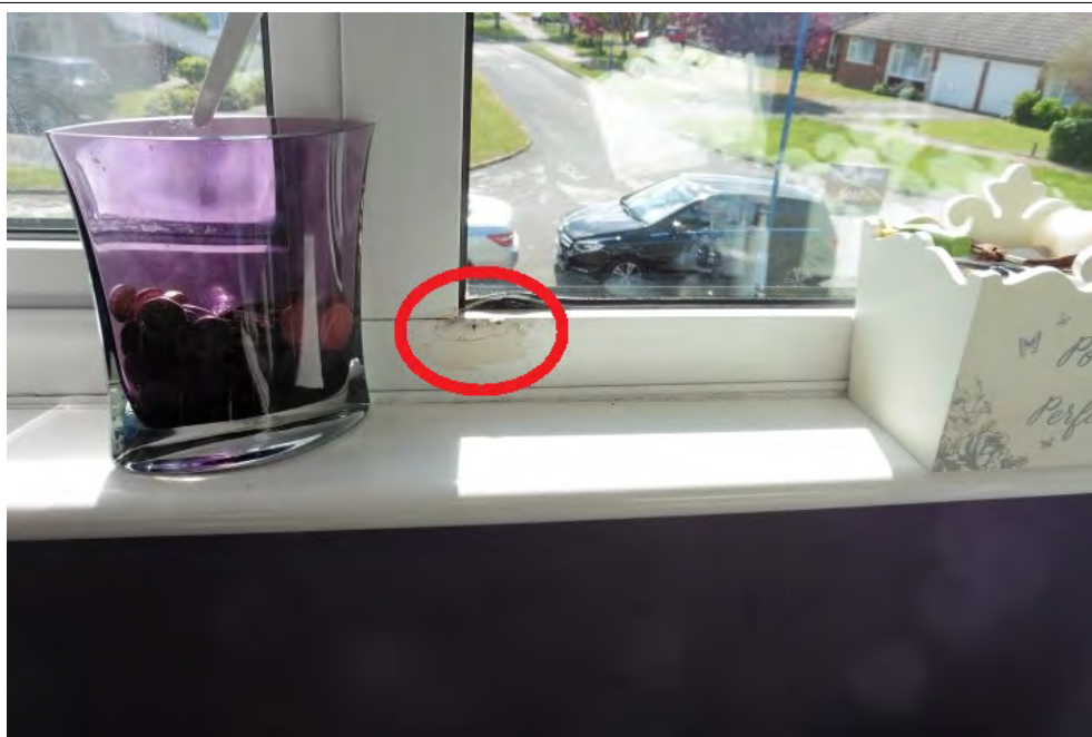
Damage to frame and seal in bedroom 1
