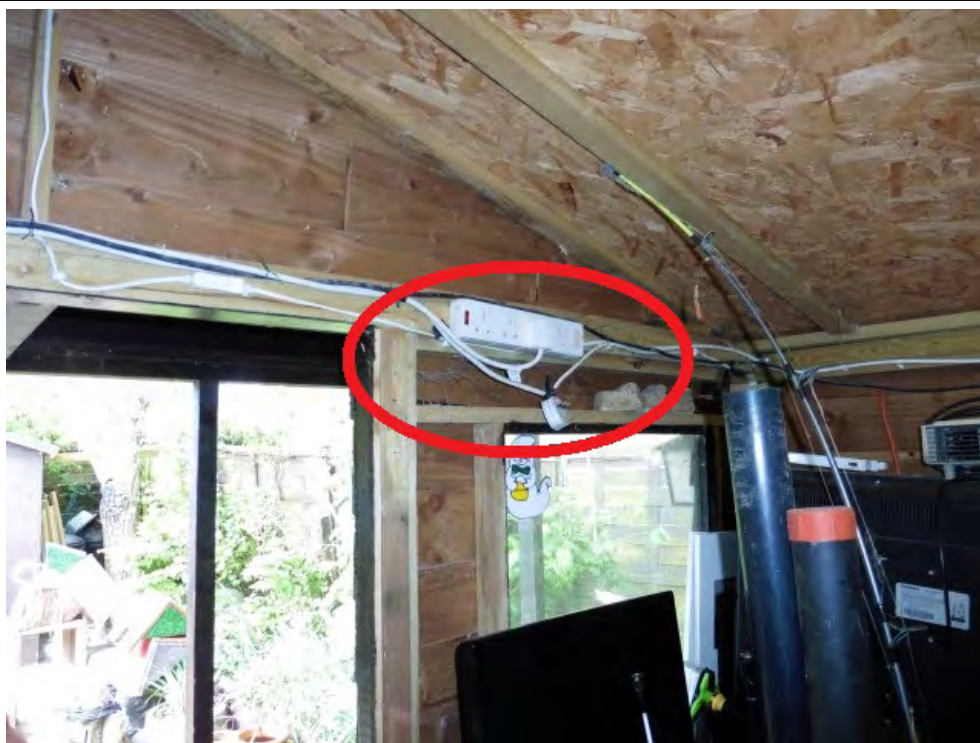
Poorly managed wiring in shed 4
